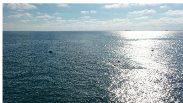
Figure 1. (a) First modules of the offshore floating solar array of Oceans of Energy installed nearshore in the Dutch North Sea in 2019; (b) Sixty-four (64) interconnected modules creating a floating farm with one-third the size of a football field, operational 12 km offshore from The Hague, the Netherlands since 2020. Farm will be expanded to 1 MW-size in 2023
