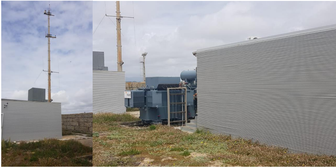
Figure 5 – Electrical grid connection substation and support station at Aguçadoura site
